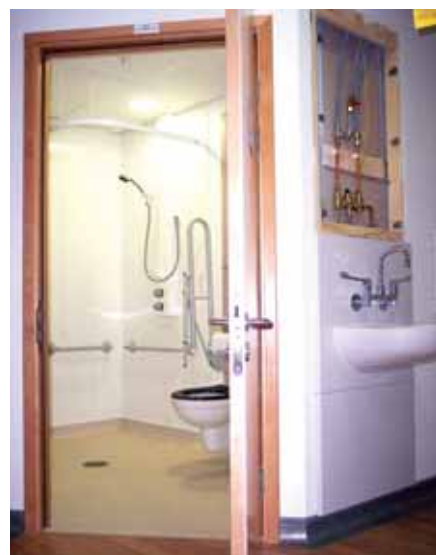
Top and above: Hygienik fitted wall linings in over 180 assisted shower rooms in Lewisham Hospital, South London
